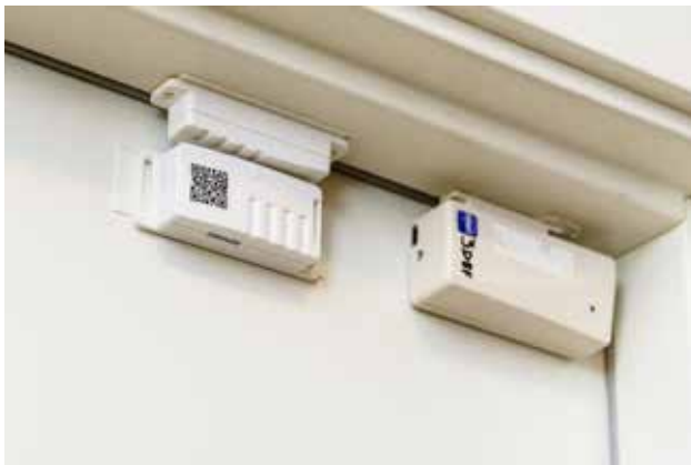
Simple door sensors for data collection in Halmstad Intelligent Home.
